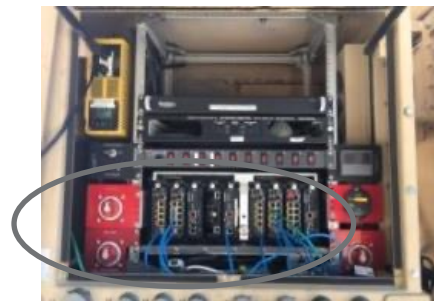
PacStar NOTM Vehicle Installation
